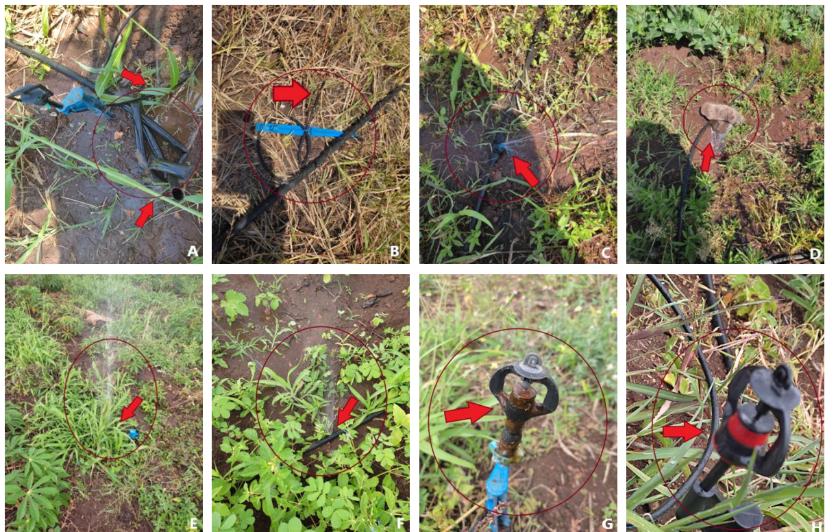
A – Leak at the end of the line caused by improper closure; B – Failure to replace the emitter in the cultivated area, with a simple interruption of water flow in the microtube; C – Leak in a faulty line valve; D – Leak in a lateral line covered by stones; E – Leak at the connection between the lateral line and the microtube of the micro-sprinkler; F – Leak resulting from a cut in the lateral line; G – Total clogging of the micro-sprinkler with easily visible causes; H – Total clogging of the micro-sprinkler with no apparent visible causes.
